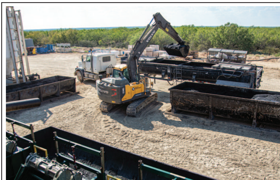
In the Eagle Ford and other shale plays, operators are implementing closed-loop systems to successfully drill long laterals while simultaneously minimizing waste and reducing environmental impacts. Closed-loop solutions encompass drilling fluid products, state-of-the-art solids control equipment, and haul-off and disposal services.
