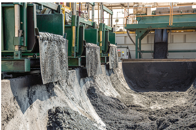
Fig. 2. The first step of the mud cleaning process is separating the cuttings from the mud coming directly from the wellbore.
